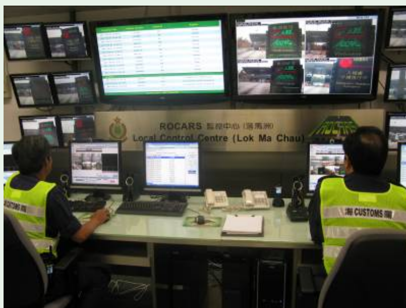
ROCARS Local Control Centre at Lok Ma Chau Control Point.
