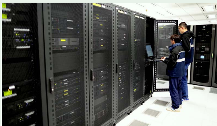
Data Center staff conducting system maintenance checking on computer servers in Customs Headquarters Building.
