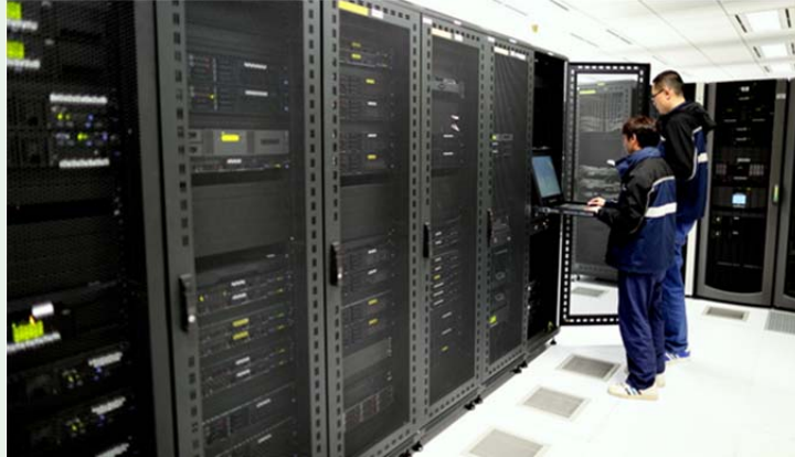
Data Centre staff conducting system maintenance checking on computer servers in Customs Headquarters Building
