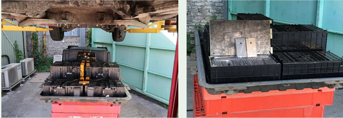
Mobile phones in a secret space in the altered battery compartment of an electric vehicle
