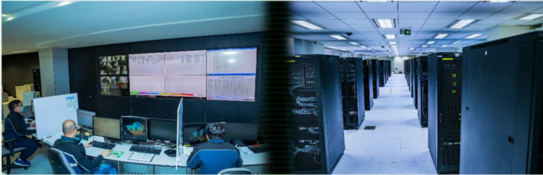
Data Centre staff conducting round-the-clock monitoring on computer servers in Customs Headquarters Building
