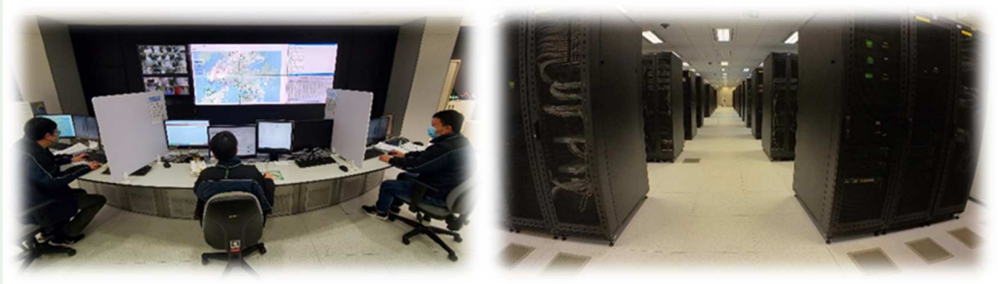
Data Centre staff conducting round-the-clock monitoring of IT Infrastructures
