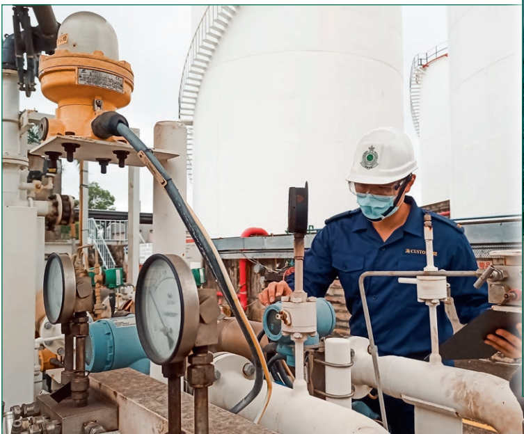
A Customs officer conducted compliance check at oil depot.
